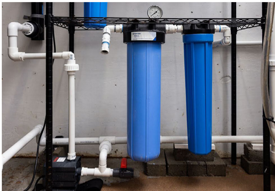
Bag filter and cartridge filter housing set up
