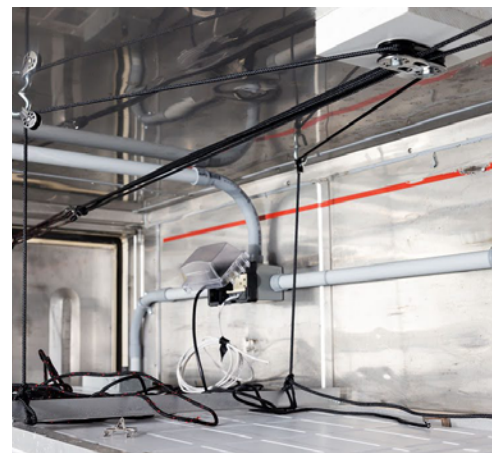
From left to right: Dimmable light, frame, ceiling suspension
